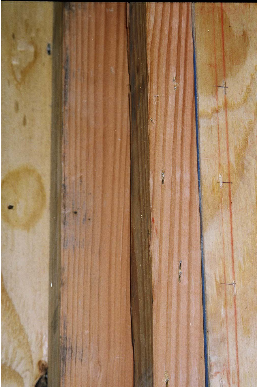
Photo 4: View of stud with staple legs sheared after flexing to form a \frac{3}{4} inch slot. The adjacent panel shows \frac{7}{16} inch staple crowns at 3 inches on center with no visible sign of distress.
